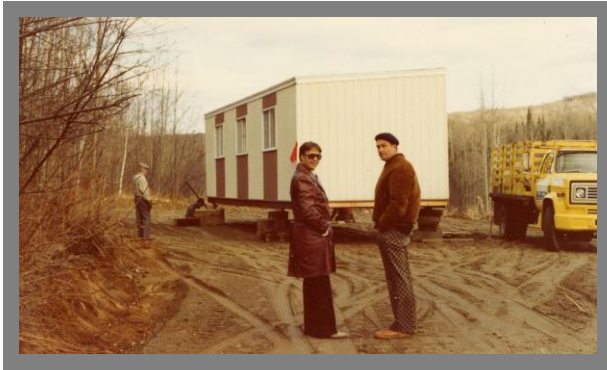
Charlie Olmsted, right, supervising installation of the first half of the building, November 1978
